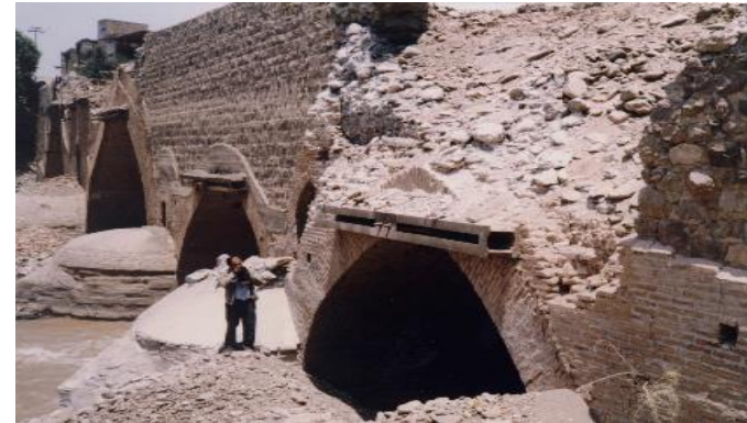
Physical damages to transportation network infrastructure
